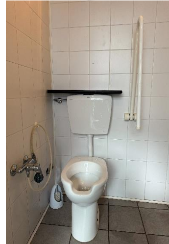
343 toilets with grab bars
